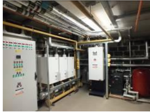
Boilers in Plant Room
